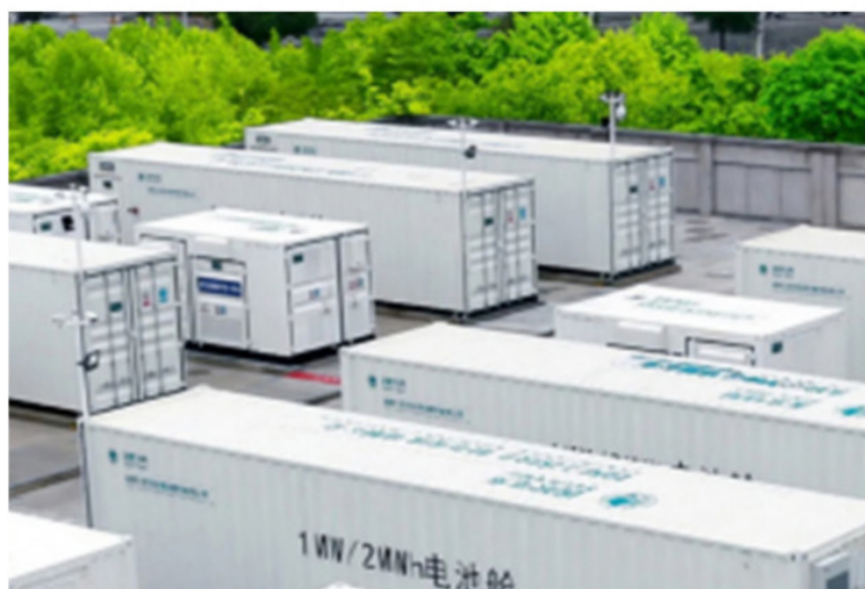
储能 Energy storage
