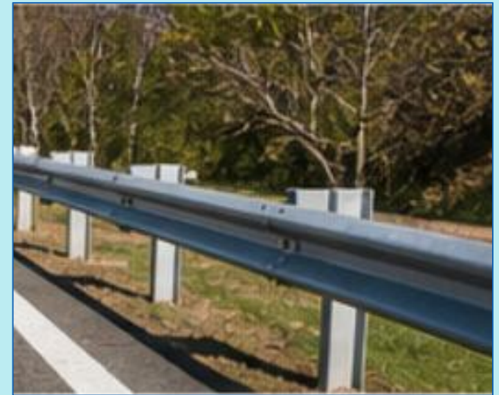
OS-T06 W-beam Guardrail
