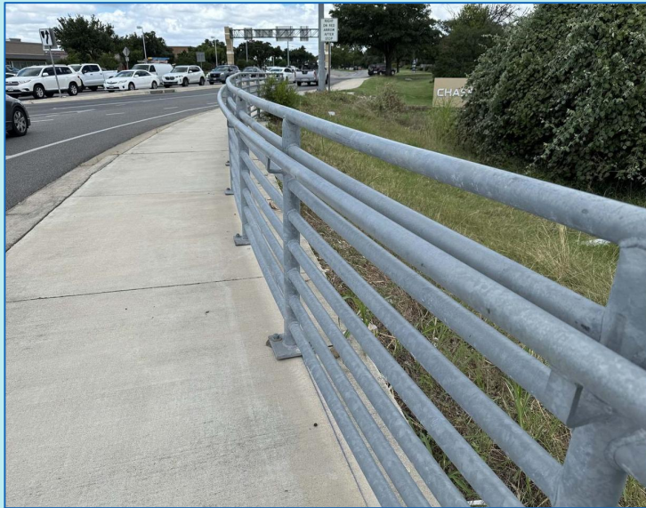
OS-T13 Pedestrian Guardrail
