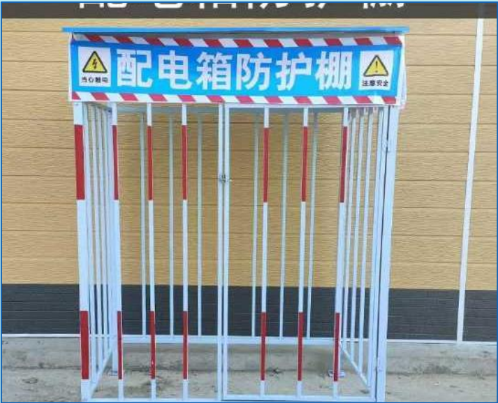
Y088 Distribution-box Shelter
