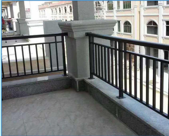
Y052 Zinc-steel Balcony Guardrail
