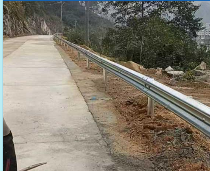
T032 W-beam Guardrail
