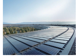
Factory Solar System
