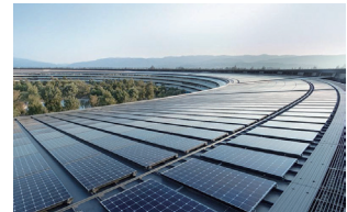
Factory Solar System
