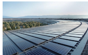
Factory Solar System
