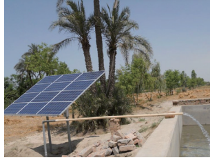
Solar Pump System
