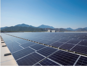
Solar Energy Storage System
