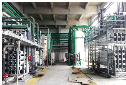
13,000 m 3 /day MMF+2pass RO+MB Boiler Water in Shandong Product water: >10 MΩ
