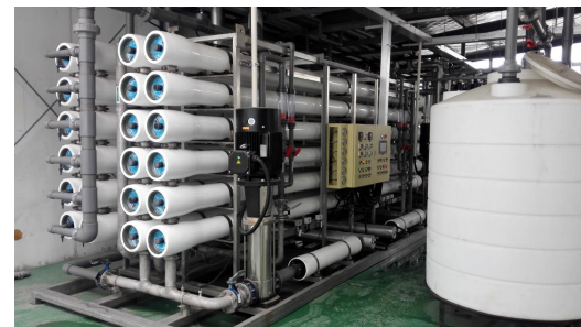
BWRO 2,000 m 3 /day · SAS Industrial process water
