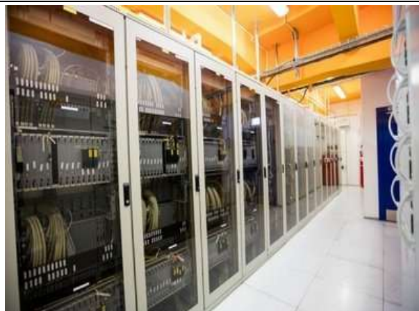
DCS 中控系统 DCS central control
