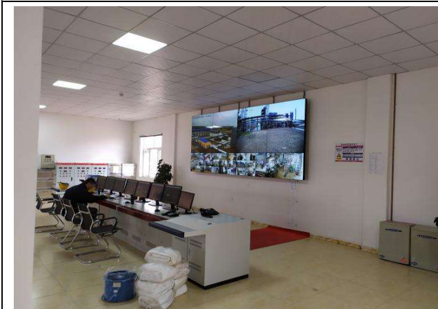
DCS 中控系统 DCS central control
