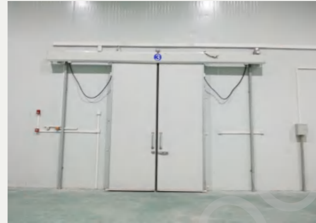
Electric sliding door
