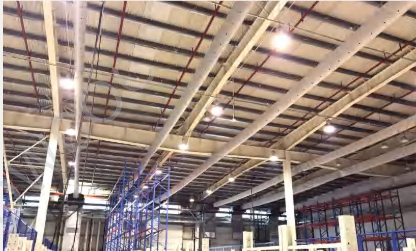
10000 tons cold chain logistics cold storage project
