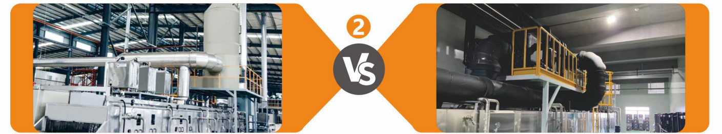
普通前处理废气装置 Ordinary pre-treatment exhaust gas device
