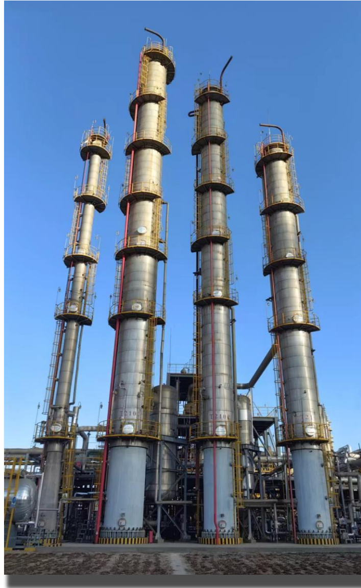
Stainless steel tower
