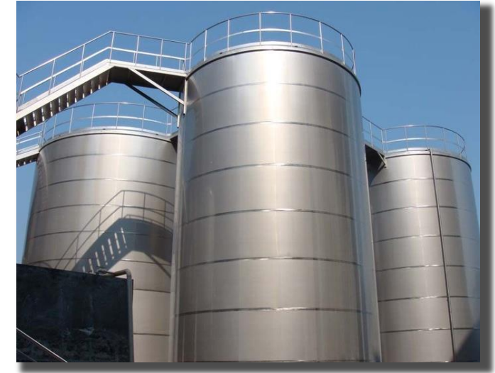
Sanitary vertical storage tank
