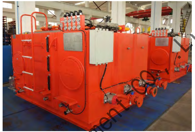
金沙江金沙水电站液压系统 Hydraulic system of Jinsha River Jinsha Hydropower Station
