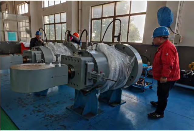
文登导叶接力器 Guide vane servomotor of Wendeng pumped-storage power station
