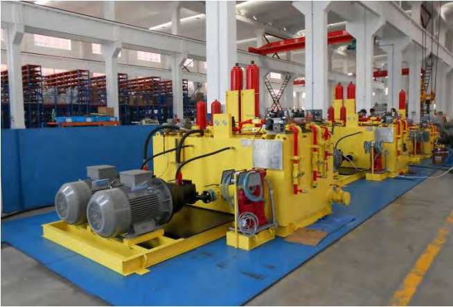
喀麦隆 隆潘卡尔水电站 液压系统 Hydraulic System of Kamailong Pankar Hydropower Station
