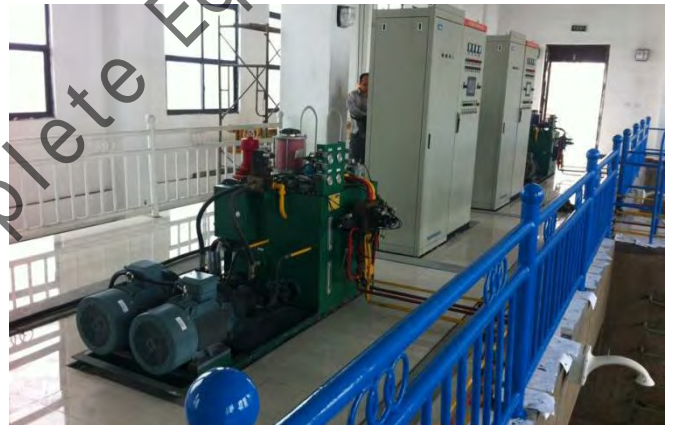
南水北调中线工程液压系统 Hydraulic System of the Middle Route Project of the South to North Water Diversion Project
