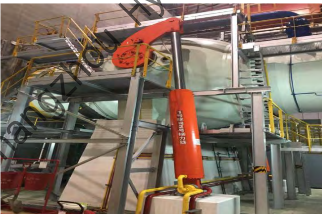
白莲河抽水蓄能电站球阀接力器 Ball valve servomotor of Bailianhe pumped-storage power station
