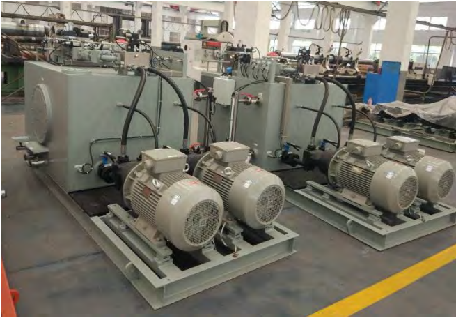
杨房沟水电站液压系统 Hydraulic system of Yangfanggou Hydropower Station
