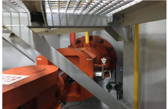
白莲河抽水蓄能电站导叶接力器 Guide vane servomotor of Bailianhe pumped-storage power station
