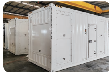
• Power Plant: 8 Units 1MW Containerized Perkins Diesel Generators
