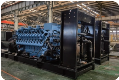
• Industrial: MTU Generator with Heat Exchangers and Remote Radiators
