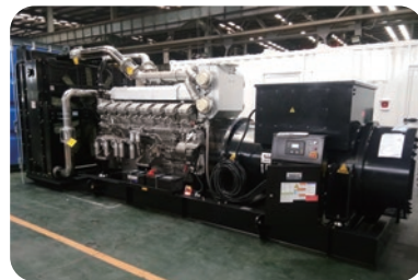
• Healthcare: 6 Units 1500KW Mitsubishi Generators
