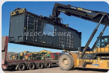
• Data Center: 2500KVA MTU Containerized Diesel Generators
