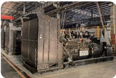
• Oil Gas: 6 Units 2500KVA Cummins Diesel Generators
