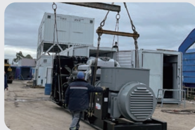
• Data Center: Standby 2500KVA Shanghai Mitsubishi Diesel Generators
