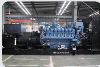
• Mining: 8 Units 1800KW MTU Diesel Generator Sets
