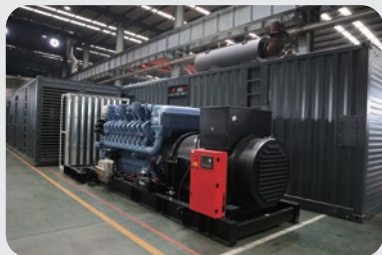
• Data Center: 1800KW Containerized MTU Diesel Generators
