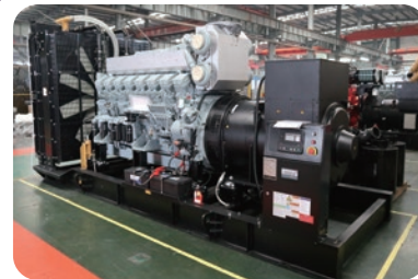
• Industrial: 6 Units 1500KW Japan Mitsubishi Diesel Generators
