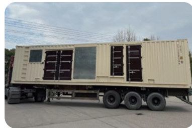
• Industrial: 4 Units 1500KW Containerized SME Diesel Generators
