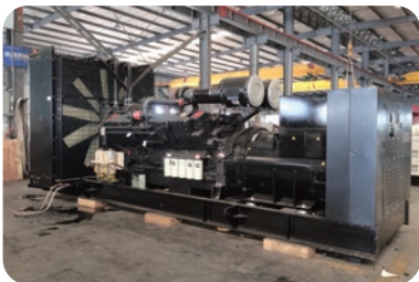
• Power Plant: 4 Units 1200KW Cummins Diesel Generators
