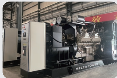
• Data Center: 2 Units 2500KVA UK Cummins Diesel Generator
