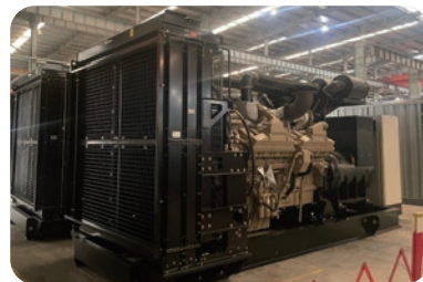
• Power Plant: 2 Units 2500KVA UK Cummins Diesel Generator Sets
