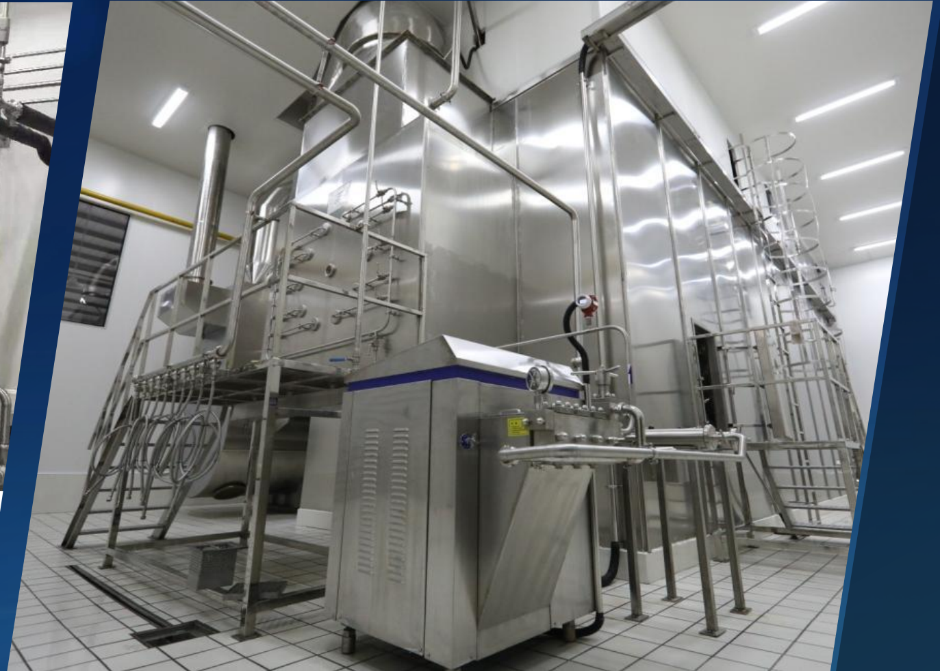
Fully Automatic Powder-Spraying System
