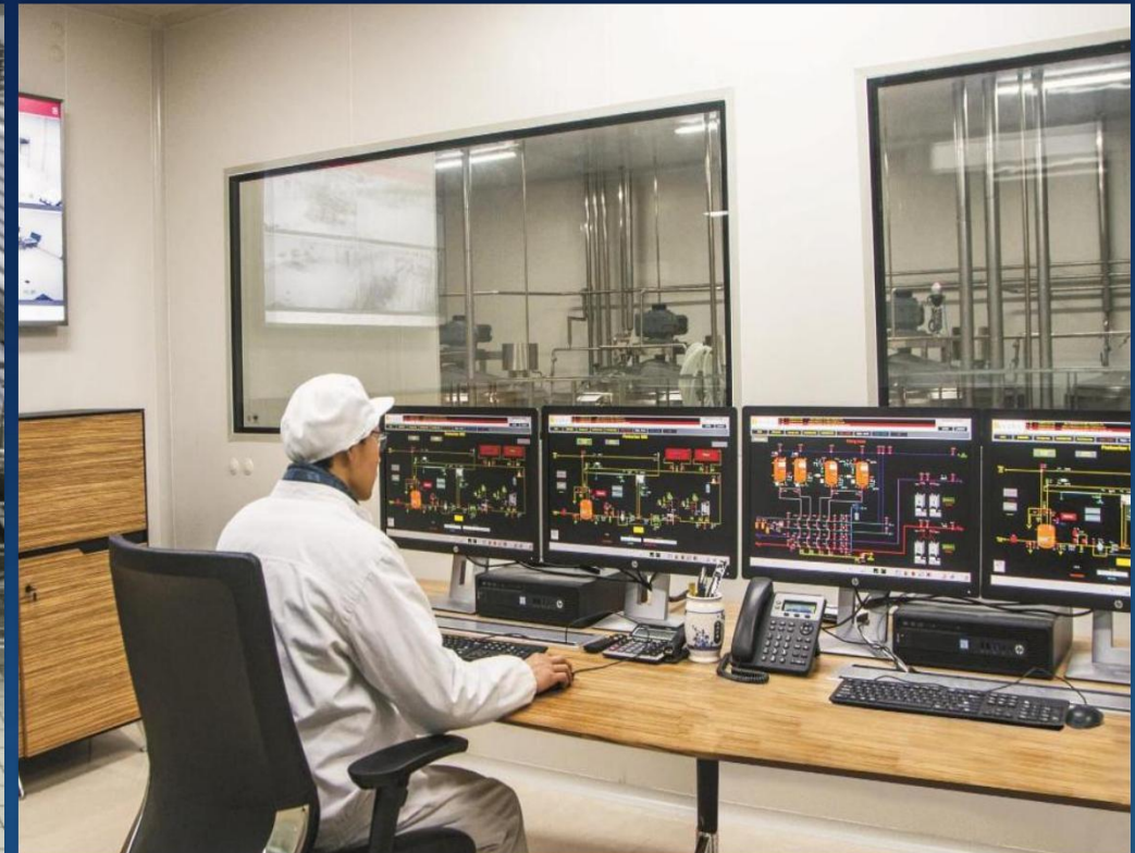
Centralized Automatic Control System
