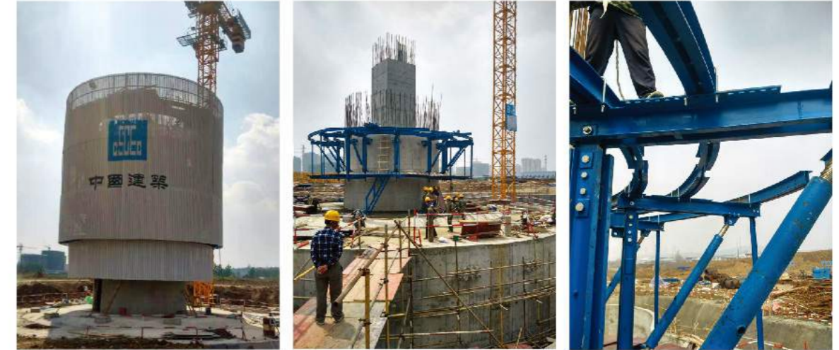
Project name: Bengbu Sports Center Landscape Tower Contractor: CSCEC, 8th Bureau Products utilized: ACS, HCB-100 (Separate Truss Type)
