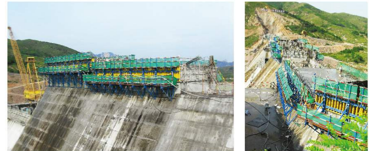
Project name: Monkey Mountain Reservoir Contractor: China Water Resources and Hydropower, No. 6 Engineering Co., Ltd. Products utilized: CB-240&CB-180 (Diagonal Brace Type)
