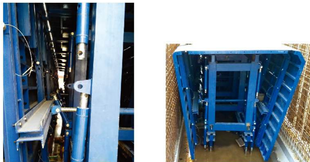
Installation of the cross brace of the top formwork and the diagonal brace of the gantry
