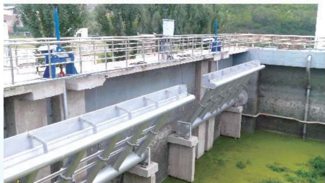
丝杆升降机用于污水处理现场 Application of screw jack in sewage treatment site
