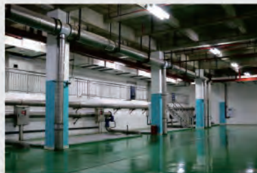
Chongqing Tangjiaqiao Wastewater Treatment Plant
