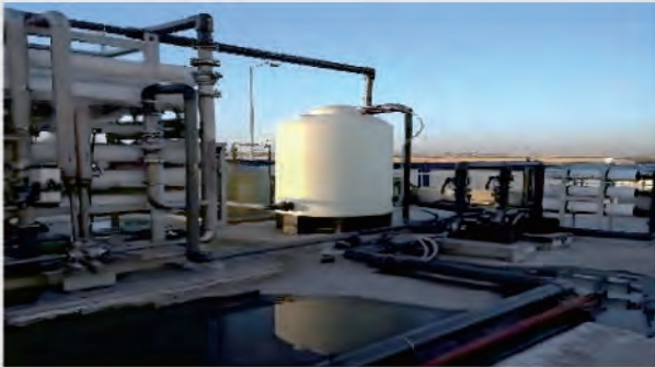
YanTai Water Egypt Seawater Desalination Project Scale: 1400 m 3 /d
