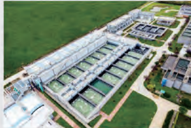
Huai'an Second Wastewater Treatment Plant
