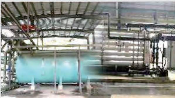
XiaoQuShanBOT Seawater Desalination Project Scale: 6000 m 3 /d
