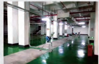
Chongqing Yuelai Wastewater Treatment Plant
