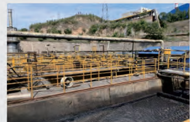
Coking wastewater treatment project of Shaanxi Coking Chemical Co., Ltd
